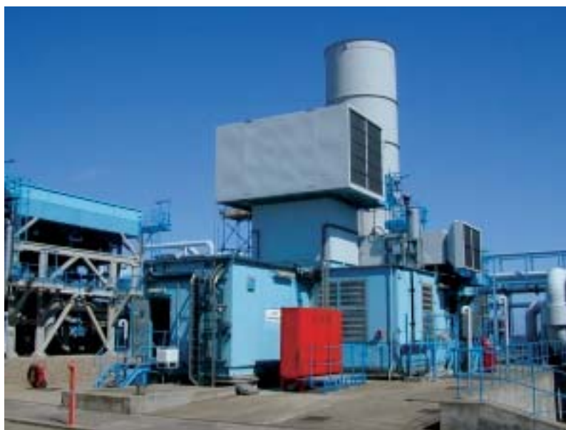
The first RB211 to be converted to DLE operates at this compressor station in the United Kingdom
